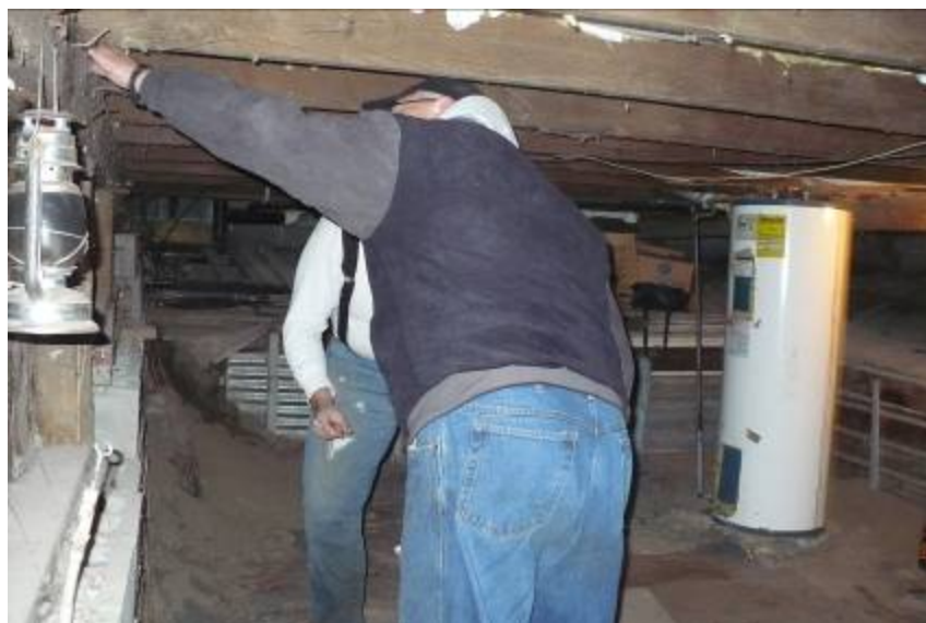
Crawl space under the house. Notice river silt on ledge to the left.
