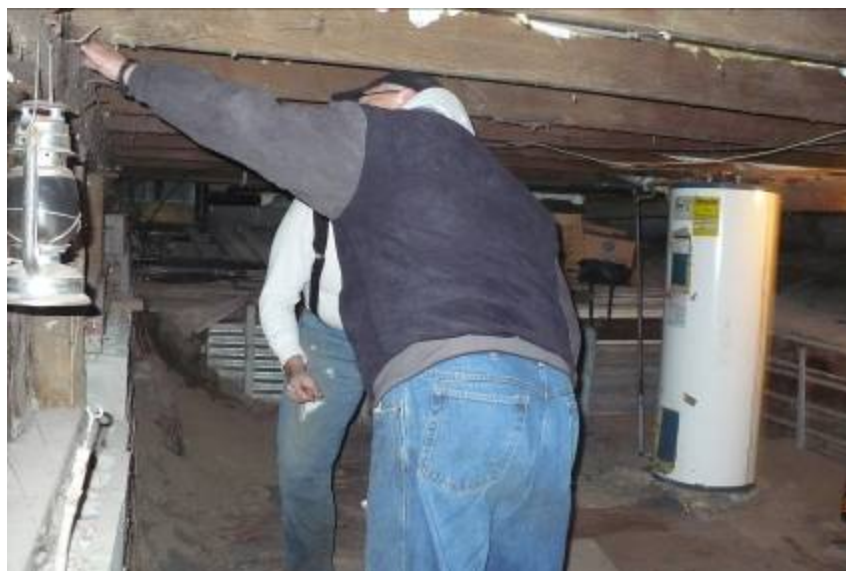
Crawl space under the house. Notice river silt on ledge to the left.
